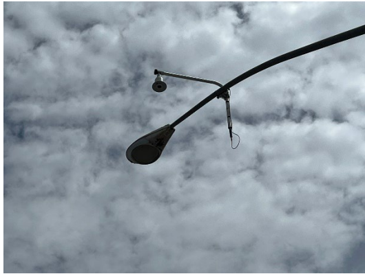
Clean CA – Median Island 11-IMP-86-PM L7.4/L7.61 Located in the City of El Centro.
