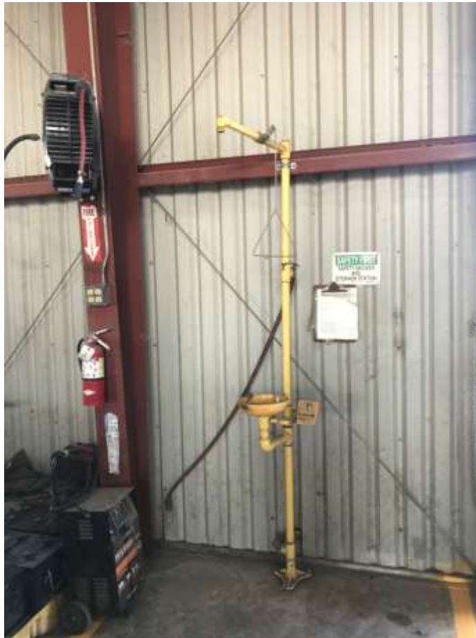
Safety eye and shower station
