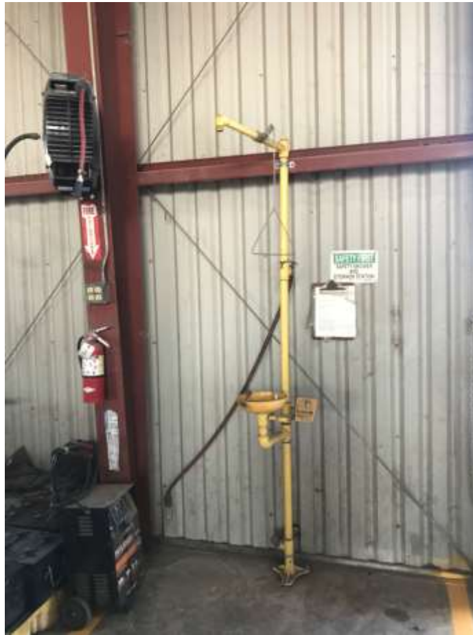
Safety eye and shower station
