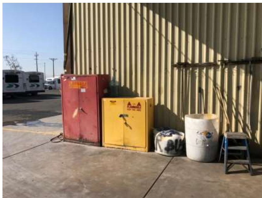
Flammable fluid storage area
