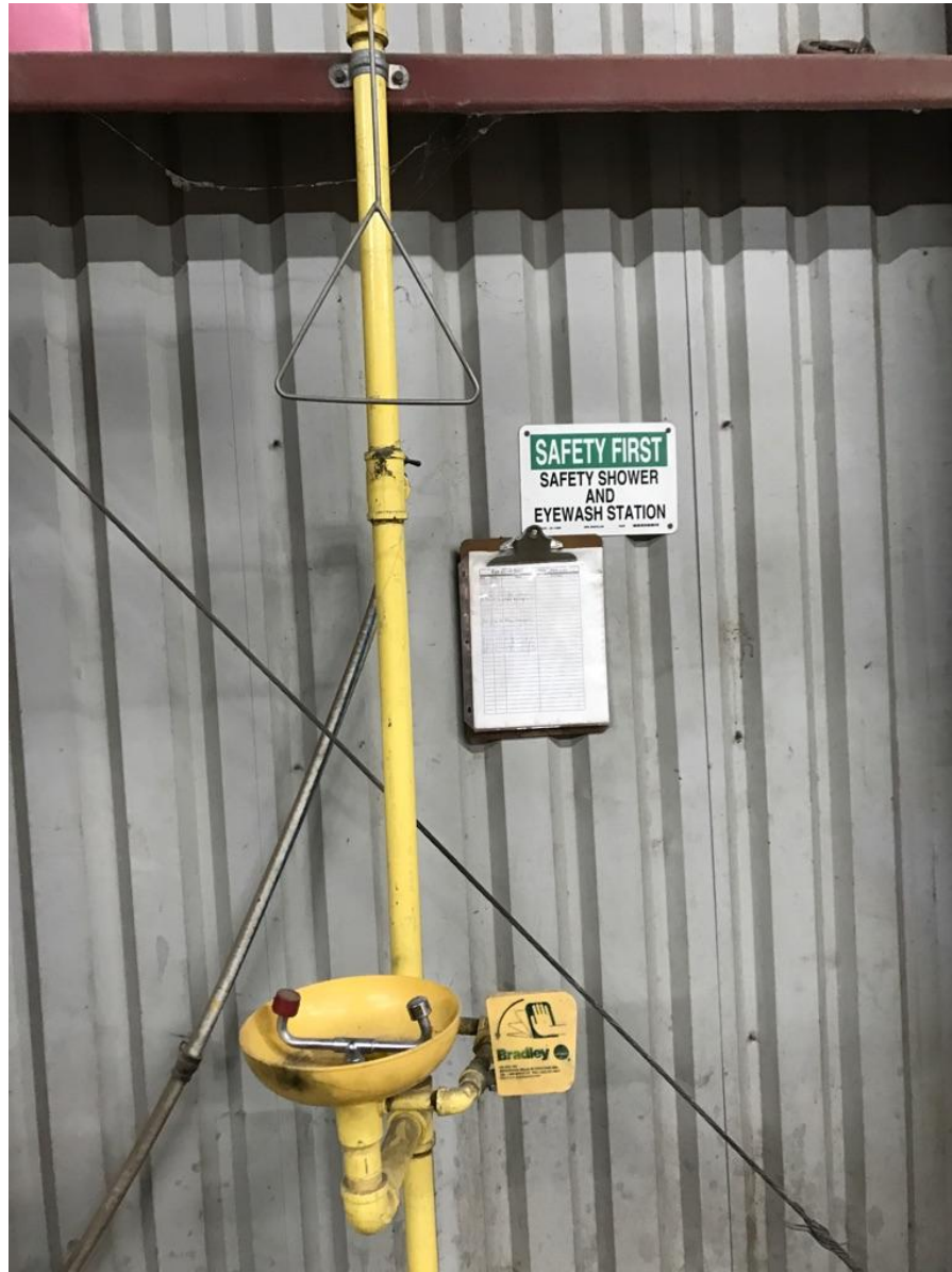
Shop safety eye and shower station
